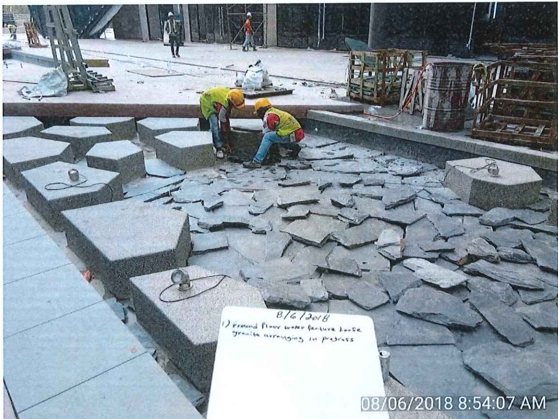
Picture 22: Loose slate and stepping stone
